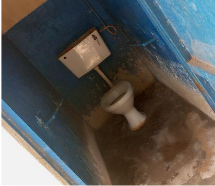
Pic 16: An old fairly modified toilet at Mbale hospital.
